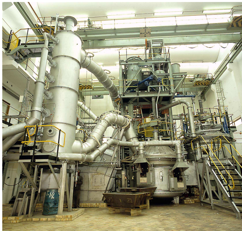
Figure 6a : Mintek DC Furnace
