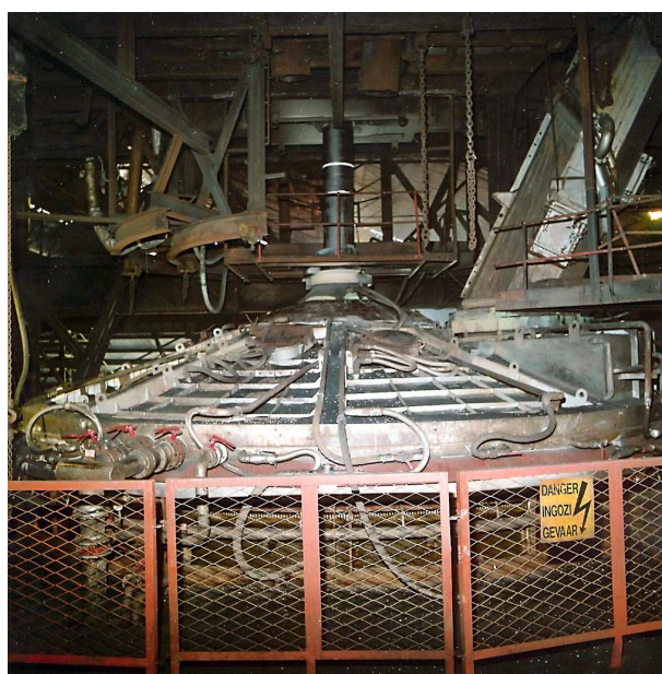
Figure 6 : Palmiet DC furnace
